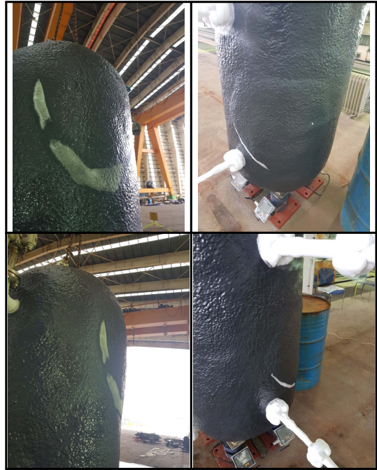
Fig. 6. Inflated insulation of re-liquefaction drum.
