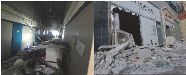
Fig. 2 Case of earthquake damage
