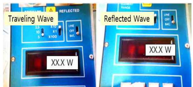
Fig. 9 Traveling and Reflected Waves of RF Cable
