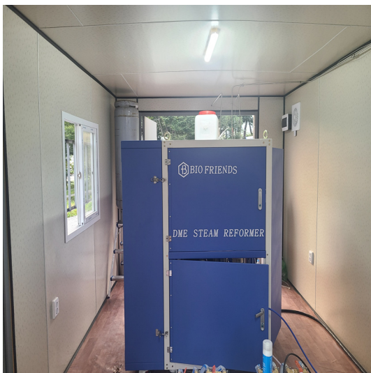
Fig. 3. DME steam reforming equipment
