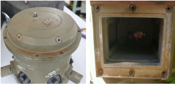
Fig. 1. Corrosion case of K000
